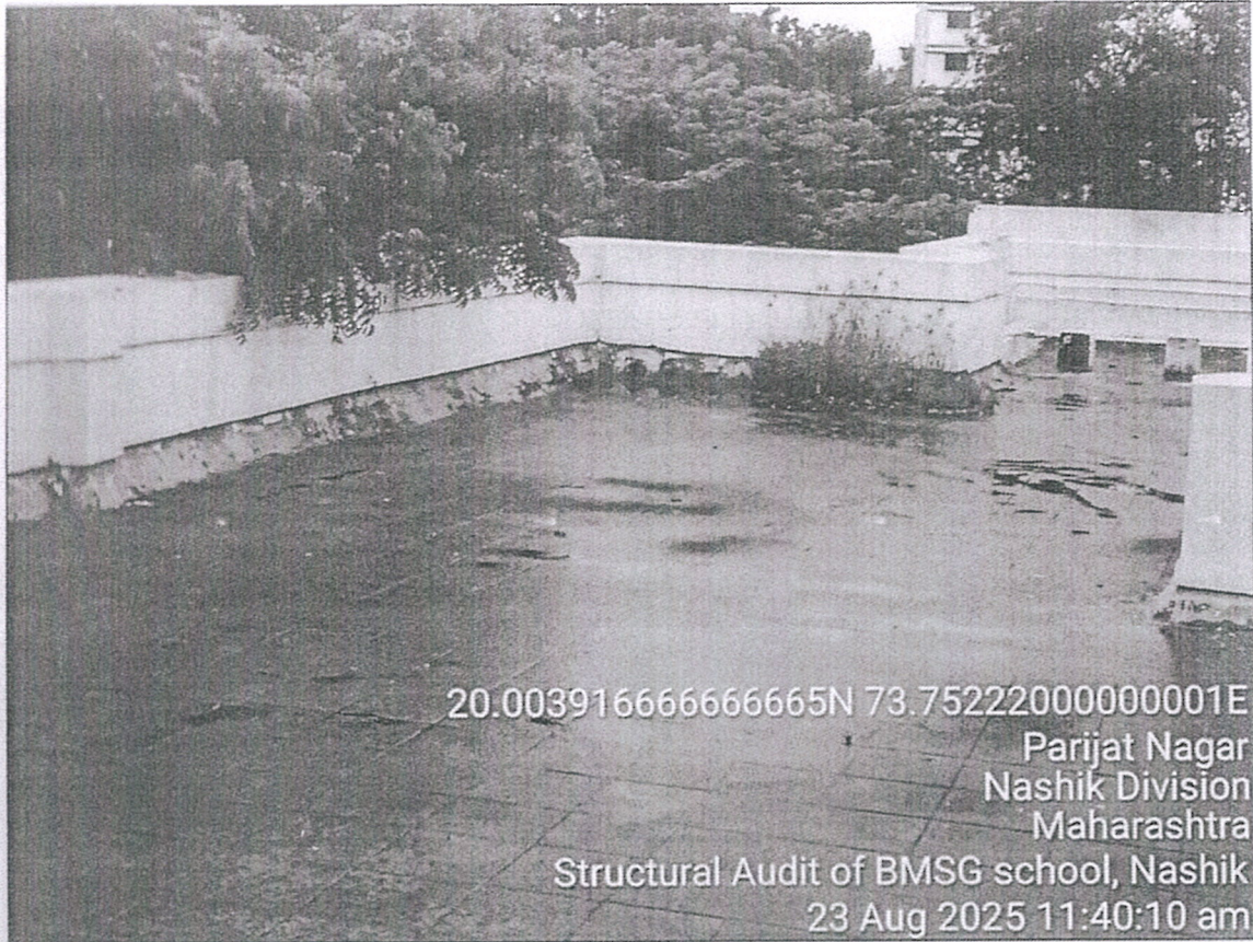
Photo No. 2- Vegetation on the terrace level at few locations.
